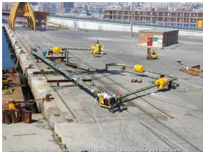
Courtesy of Dan Fjellroth | An example of a quayside SIT with a complex pipe spool piece.
